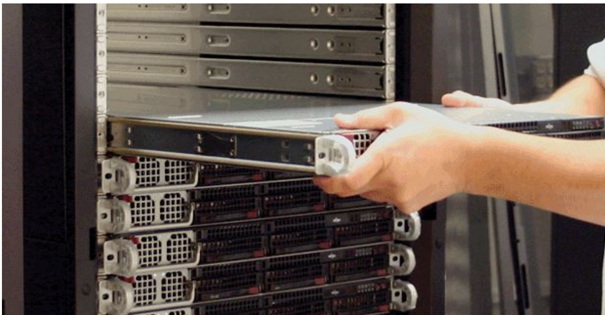
Figure 3. A rack of servers
