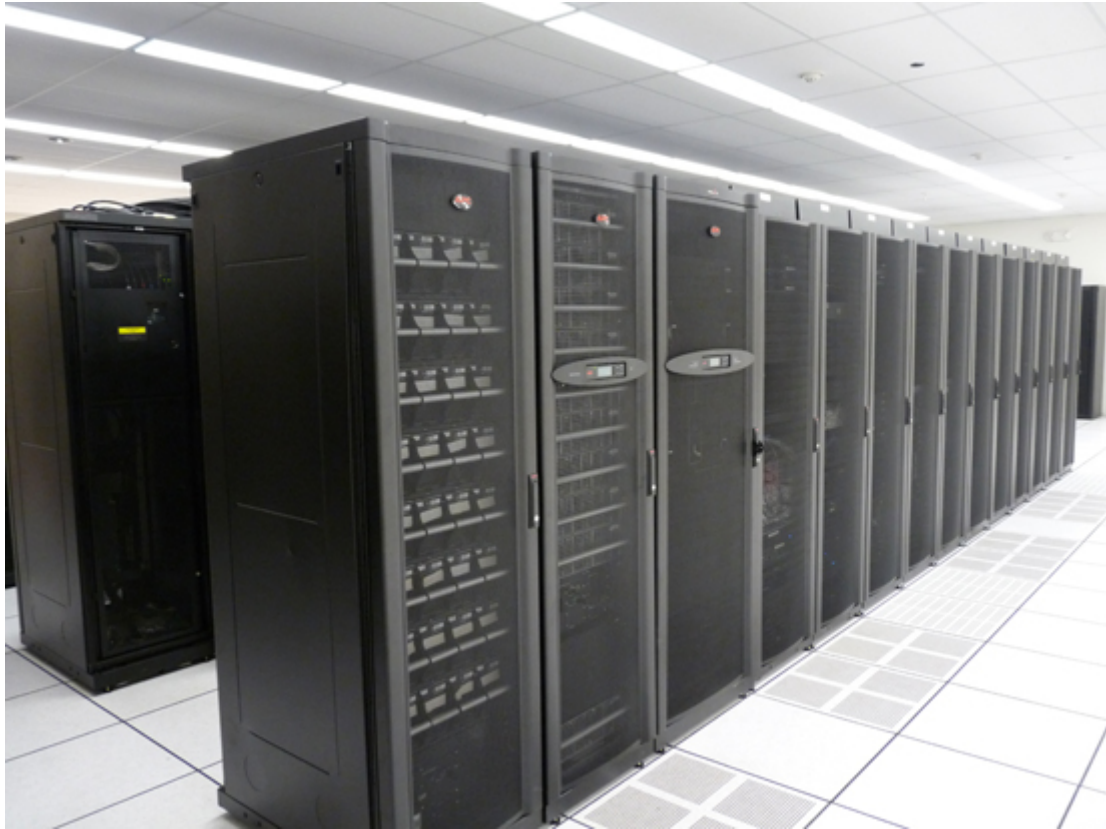
Figure 4. A data center
